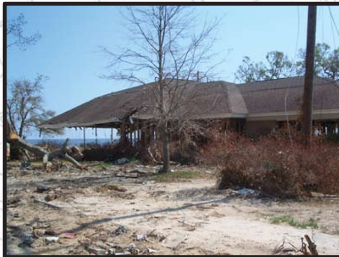
Our Lady of the Gulf Parrish Rectory Destroyed Barter & Associates is Designing a Replacement
