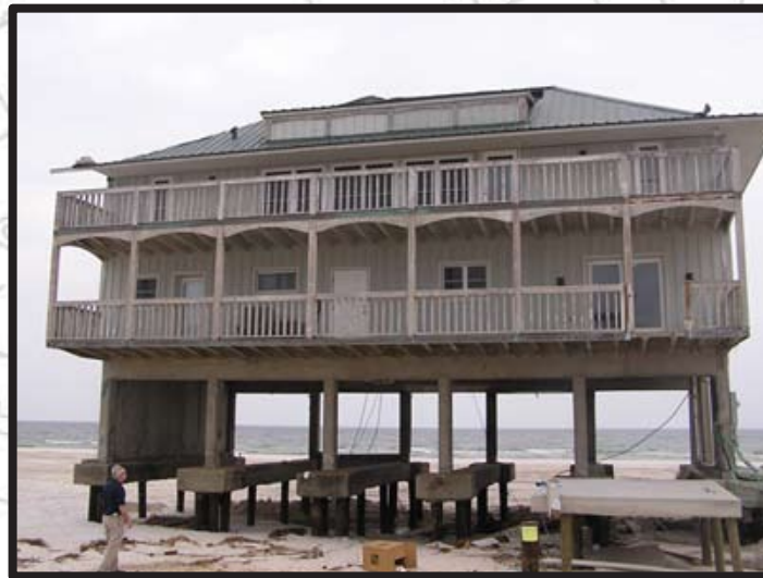
Residence Undermined by Storm Surge
